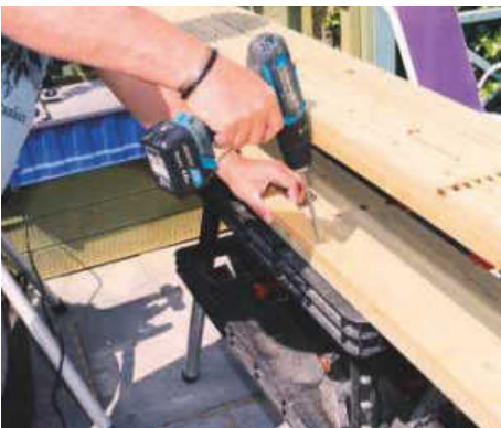
STEP 13. Battens are screwed inside at the bottom, ready for the base
